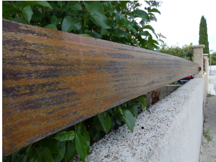
Vertical enclosure on a low wall without a guard rail, Teyran (France).
