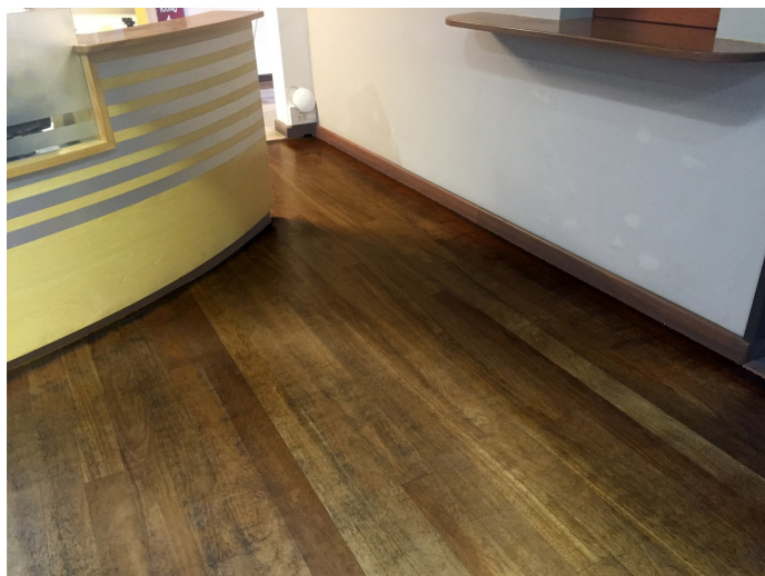
Floor at the offices of Fibres Industries Bois, Saint Paul, La Réunion (France).
