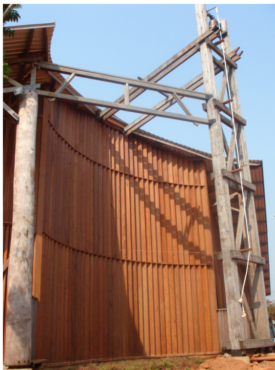
Belfry and sawtooth cladding in Mukulungu and posts in Tali – By J.Y. Riaux, Mindourou (Cameroon).
