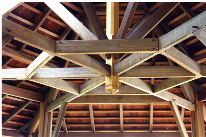
Traditional roof structure made of Basralocus (shingles in Wallaba) - Kourou (French Guiana).
